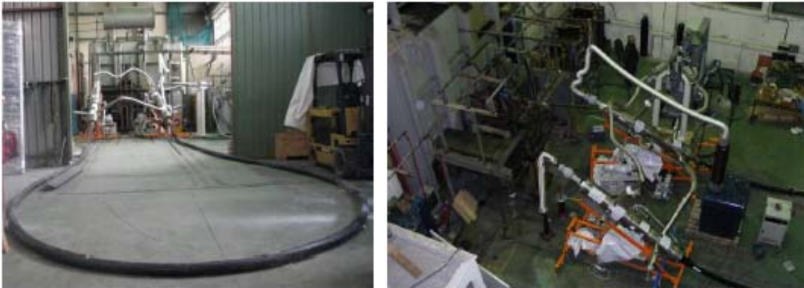
Fig. 2. Installation of the HTS cable at LABEIN TECNALIA for short-circuit and dielectric tests. Left: 30 m long functional model cable. Right: Overview of terminations and connections for the dielectric tests.
