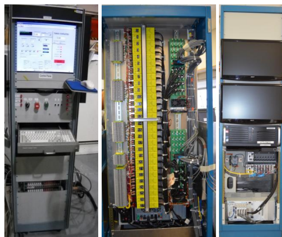
Fig. 11. Part of the advanced quench detection electronics system that was specifically developed (a) to have a high sensitivity to detect the onset of the pre-quench phase at the mV or lower level in large coils and (b) tolerate high isolation voltage (over 1 kV) for fast energy extraction.
