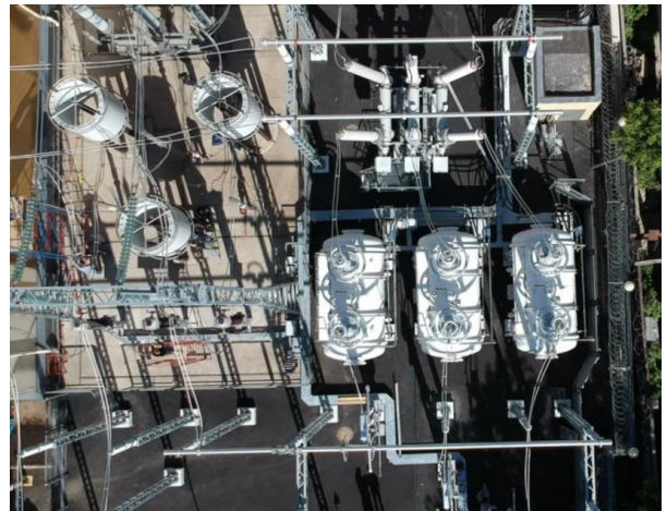
Fig. 2. Front (upper picture) and top view (bottom picture) of the 220 kV SFCL at the substation in Moscow.
