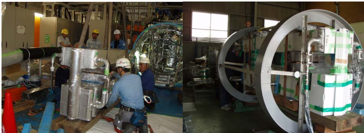
FIGURE 6. The left photo shows cutting process of the heat exchanger unit from the refrigerator. The right one shows a cleaning process of the heat exchangers in a factory.
