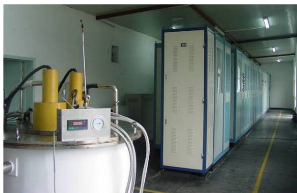
Fig. 19. The 1 MJ/0.5 MVA HTS SMES system.
