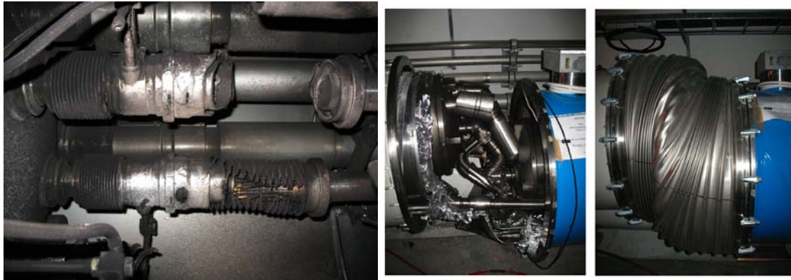
Figure 17. Pictures of the damaged zone after the incident. Left: zoom on the interconnection where the first arc happened, with vaporized cryogenic and vacuum pipes and soot deposited everywhere. Right: an interconnection between dipole (blue) and quadrupole (white) with interconnection bellow heavily deformed by displacement of the quadrupole against the dipole. Centre: the same interconnection after removal of the bellow.
