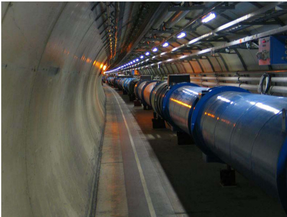
Figure 1. The superconducting magnets in the LHC tunnel
