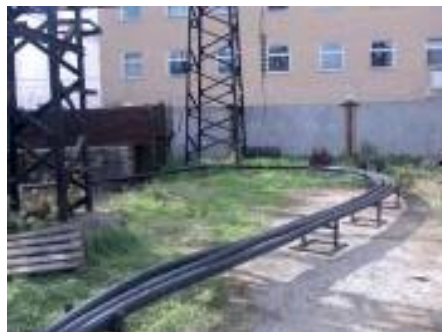
Fig. 17 (b). Three phases of the 200m long cable installed on the grounds of the test site.
