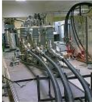
Fig. 17 (a). Terminations of the 200 m long cable installed at the test site in R&D Center for Power Engineering.
