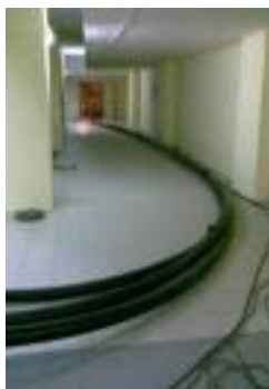
Fig. 13 (b). The 30 m long three-phase cable at the test facility.
