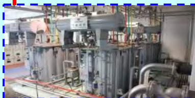
Power Supply System
