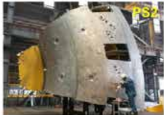
PS2 ◀ Welding of inter-modular & centering keys of inner shell of upper segment (PS2)
