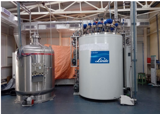
Liq. Helium plant installed at VECC Kolkata
