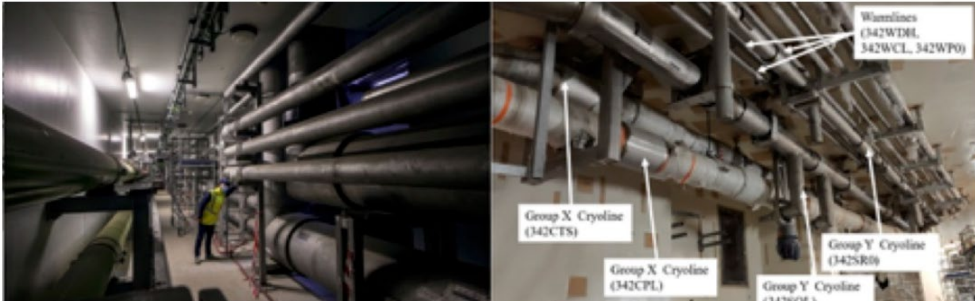
Cryolines and Warm Lines manufactured by INOX CVA under Installation at ITER, France
