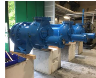
Maintenance of LHC compressors
