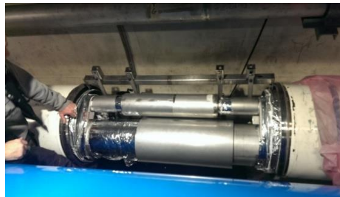
Repair of metallic compensator in the LHC cryogenic distribution line during LS2 (2020)
