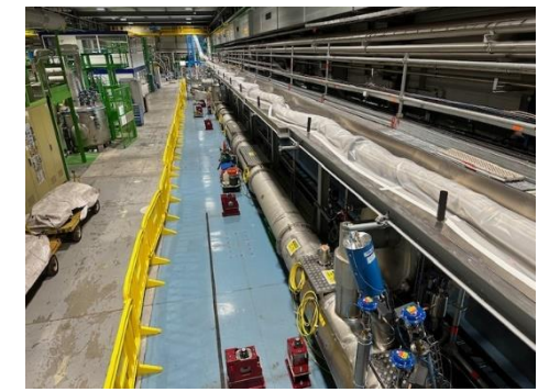
HL-LHC String: SC link and cryogenic distribution line
