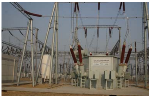
Fig. 3. A view of the 220kV/800A FCL after installation at Shigezhuang substation in Tianjin
