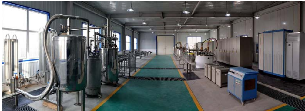
Fig. 1. A view of the superconducting power substation
