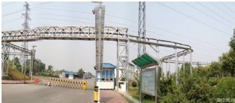
Fig. 2. The view of the 10kA HTS DC power cable after installation.
