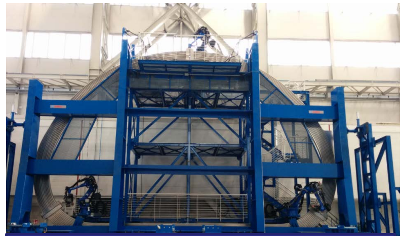
Sectors are welding by NG GTAW or LV EB (in photo GTAW welding-SIMIC)
