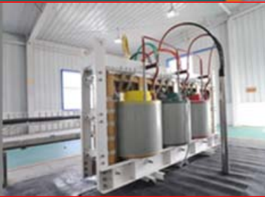
10kV HTS Transformer
