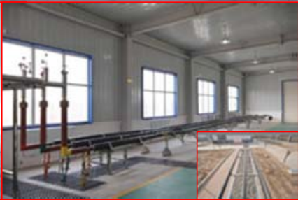
75m/10kV Power Cable
