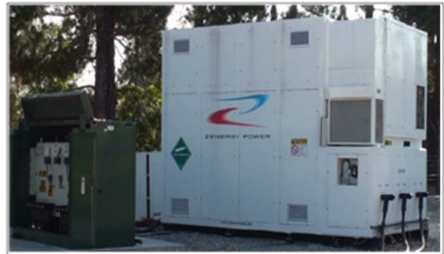
Fig. 8 – The CEC FCL installed at the SCE Shandin Substation in San Bernardino, California.
