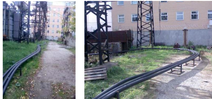
Fig. 5. The 200 m cable installed at the test facility in Russian R&D Center for Power Engineering.
