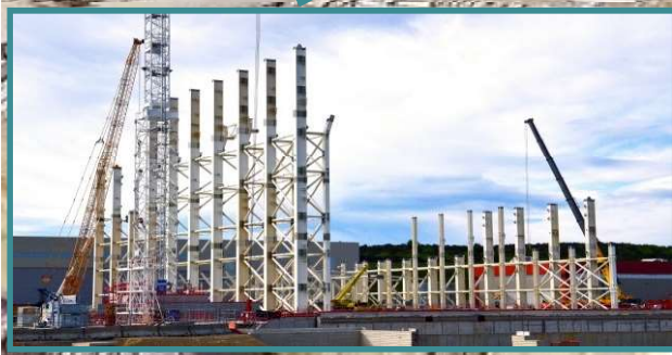
TKM Assy Hall (60 m high; to be outfitted with 2 x 750 t cranes)
