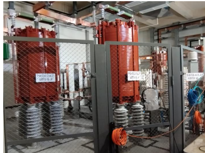
50MW AC-DC-AC substation
