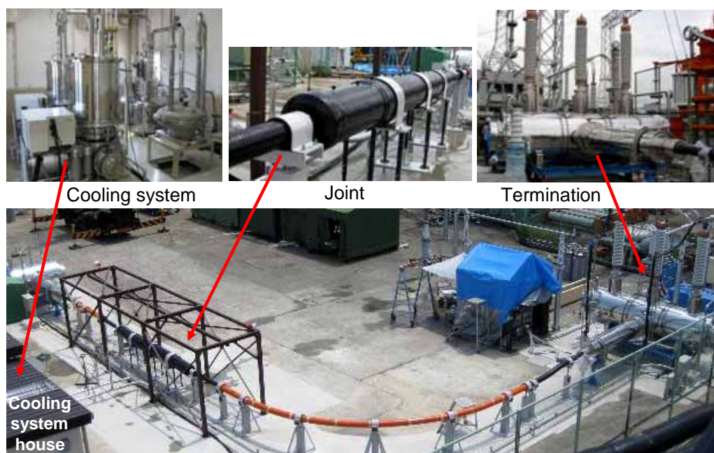
Figure 7. Cover shot of the 30-meter HTS cable system.
