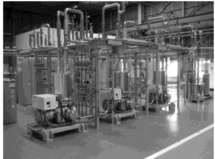
Fig. 12. Overview of the cooling system constructed at Mayekawa's factory. This cooling system has the same configuration as that for Asahi substation, though the number of refrigerator is three instead of six.
